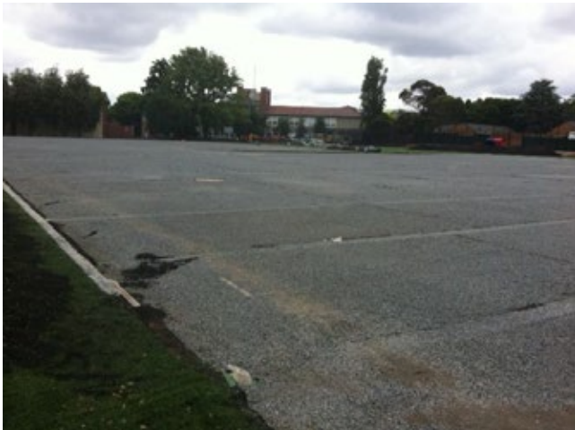
Photo 5 Ag drains to have a tendency to move after installation which impacts on the surface
