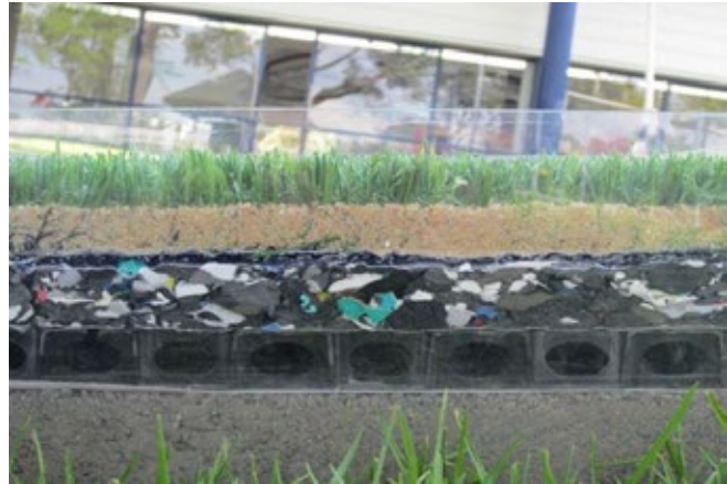
Photo 14: Example of horizontal drainage cell under shockpad (Source: Wayne Stuart - City of Swan, WA)
