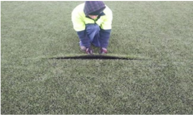
Photo 10: Example of seam failure
