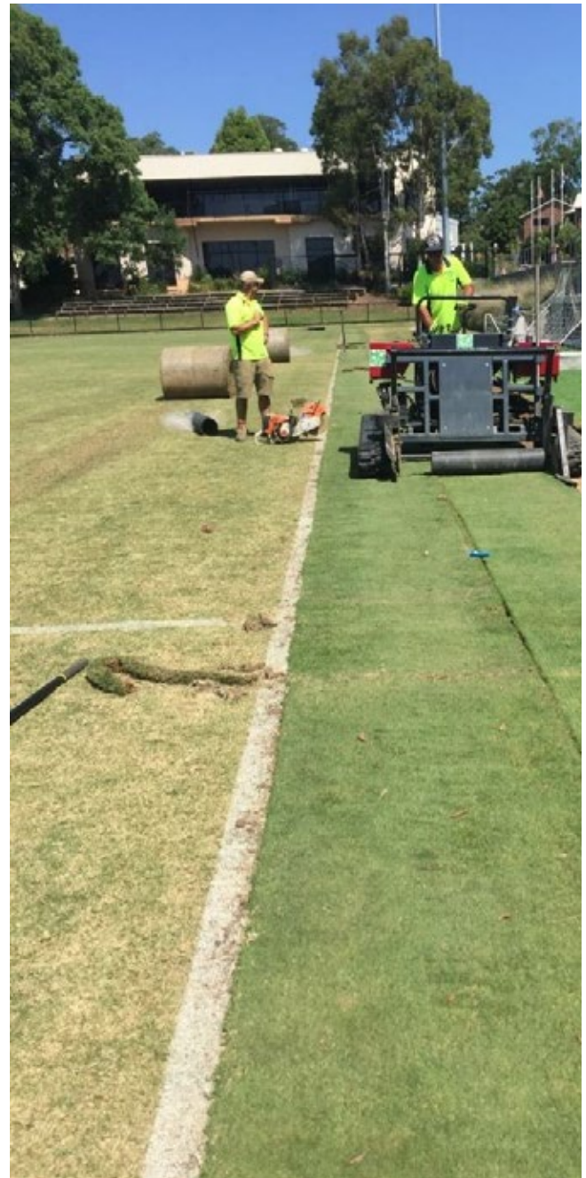
Photo 17: Lines person running lines being reinforced with hybrid technology (Source: HG Sports Turf)
